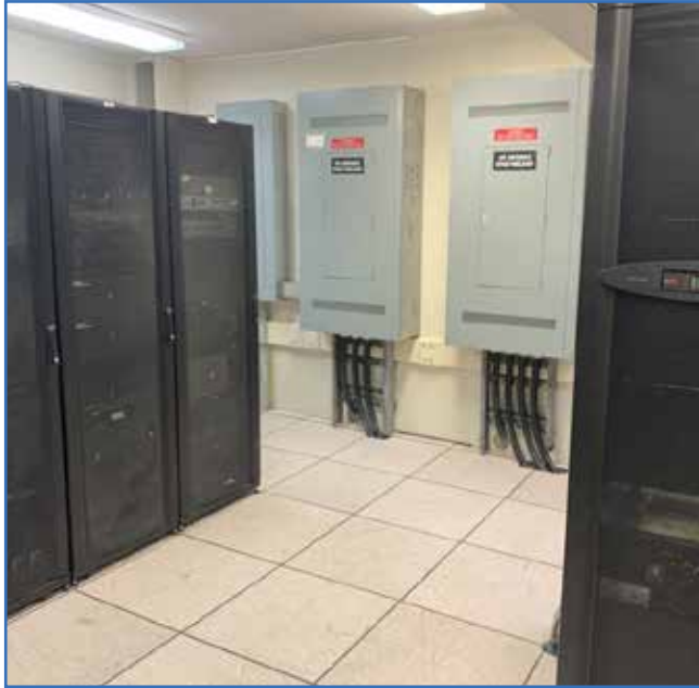
Data Centre 1 CITS New Power Infrastructure
