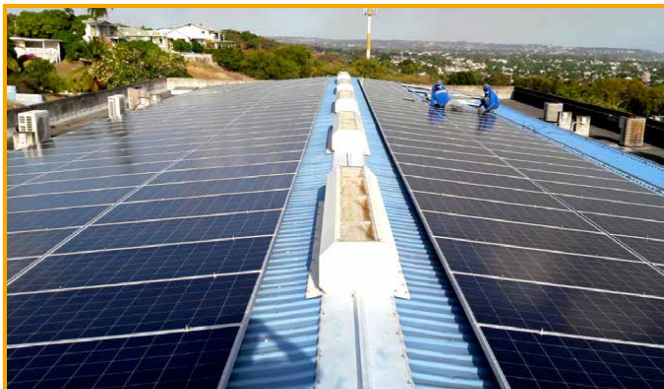
Connected solar PV system on the roofs of the Sagicor and CLICO Buildings
