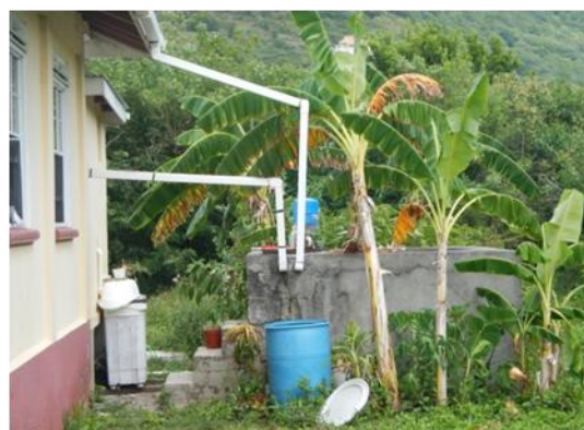
Above ground cistern with guttering system
